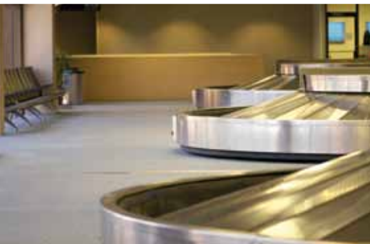
Vanderlande Industries' baggage handling system at Terminal 5 in London's Heathrow Airport is one of the most complex, innovative projects of its kind.
